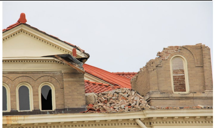
A piece of roof was ripped away over the jury room.
