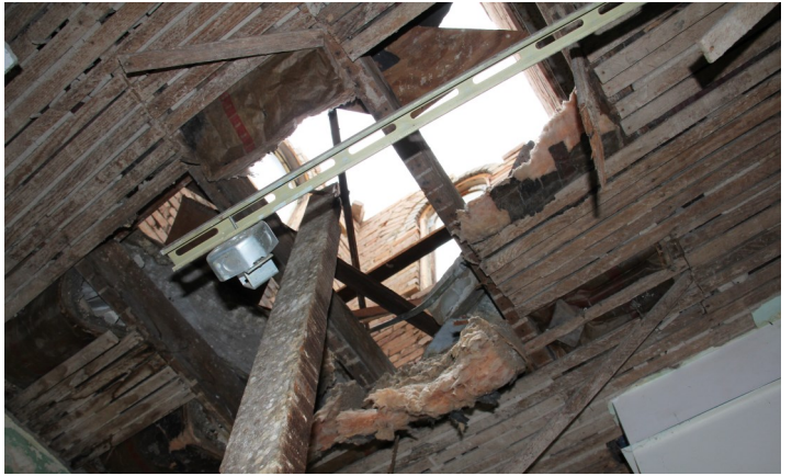
Daylight streams through a hole in ceiling above jury room.
