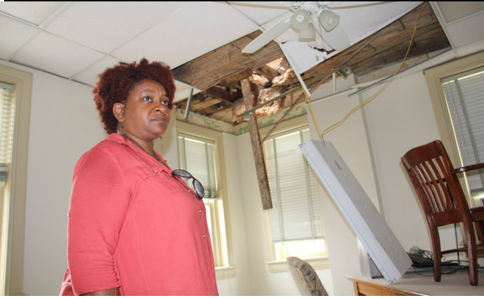
Circuit Judge Tony Terrett looks at damage in jury room.
